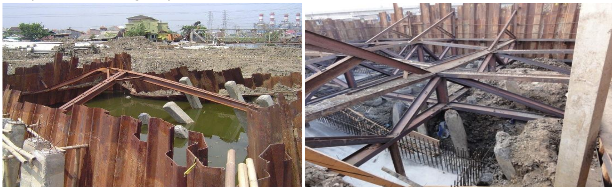
Figure 13 Left collapse of the building pit; right the new building pit.
